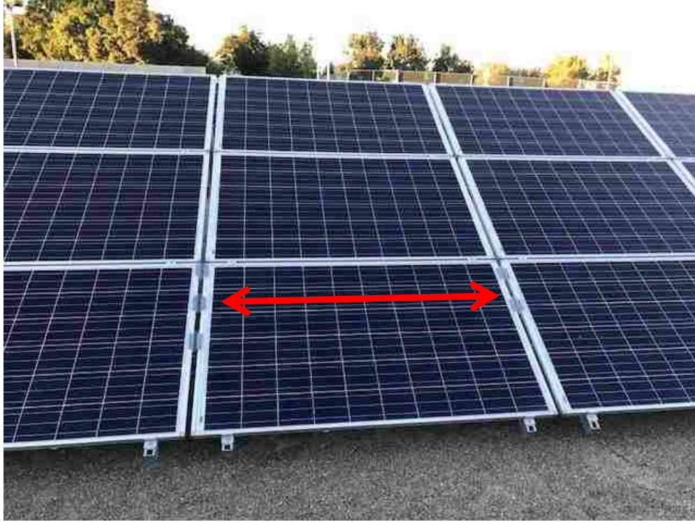
Figure 9. Tempered glass samples fixed to the solar panels to verify the amount of dust accumulated per cleaning, and the efficiency of cleaning
