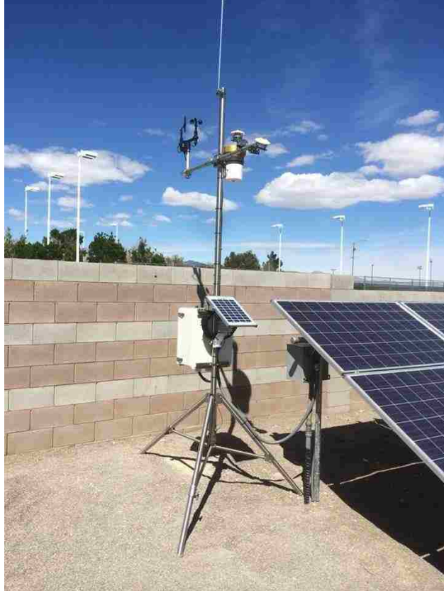
Figure 4. Weather Station installed at the City of Las Vegas West Maintenance Yard to assist in the data collection for the solar plant
