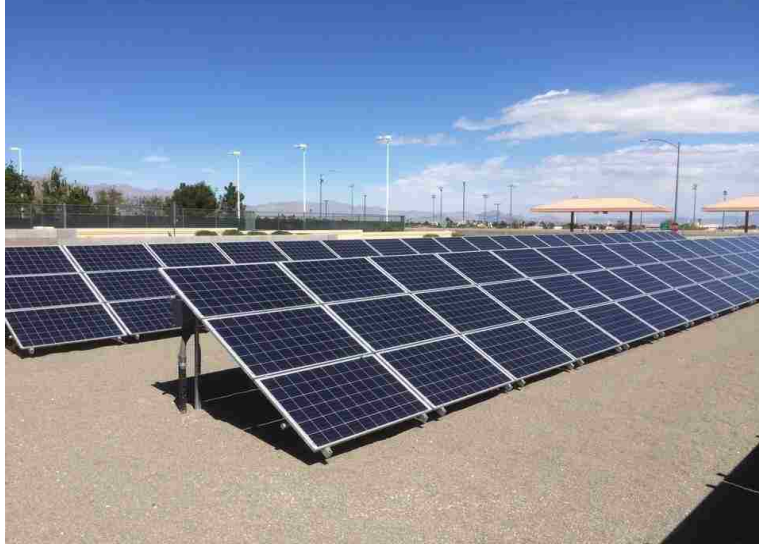
Figure 5. Instrumented 264 PV modules located at the West Maintenance Yard of the City of Las Vegas used in the study
