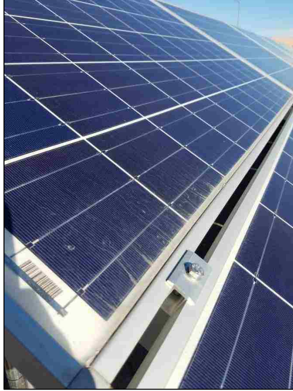
Figure 17. Presence of soiling near the edges
